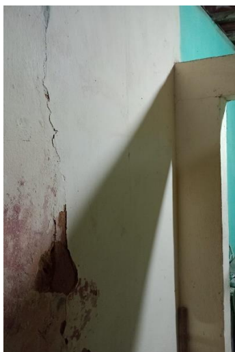
(c) Vista total fissuras
